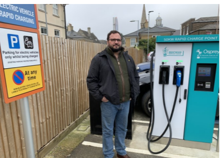
Council Leader Chris Hossack with the EV charging point installed at the town hall.
